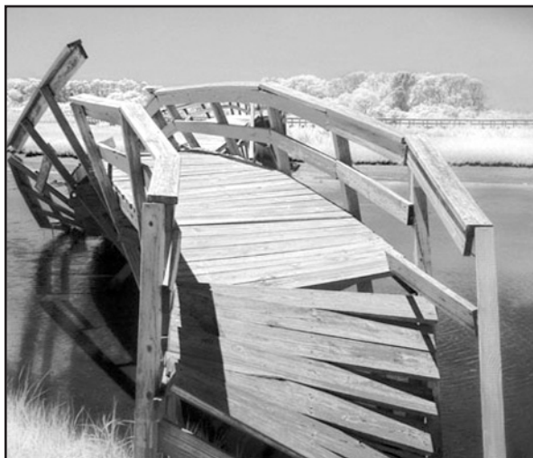
Former Watch Hill bridge, 2004, pulled up by the ice.
